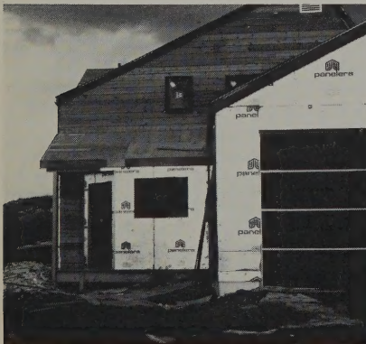
Part of a housing development, this house is a project of the students of Northwest Community College.
